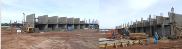
Civil Dormitory 1st Floor walling and suspended slab & Columns at NTC Kaliro
