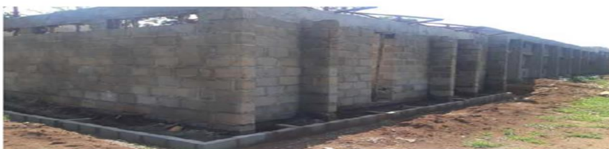
v) Building of splash apron plinth walls on washroom extension on existing dormitory, Lumumba
