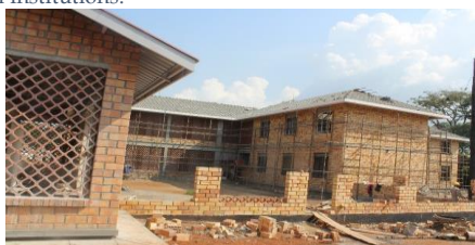
A boys' dormitory approaching completion at St. Simon Peter's Vocational Training Centre Hoima
